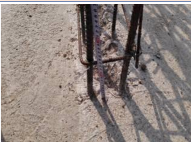
框架柱、剪力墙暗柱第一道箍筋绑 扎>50mm
