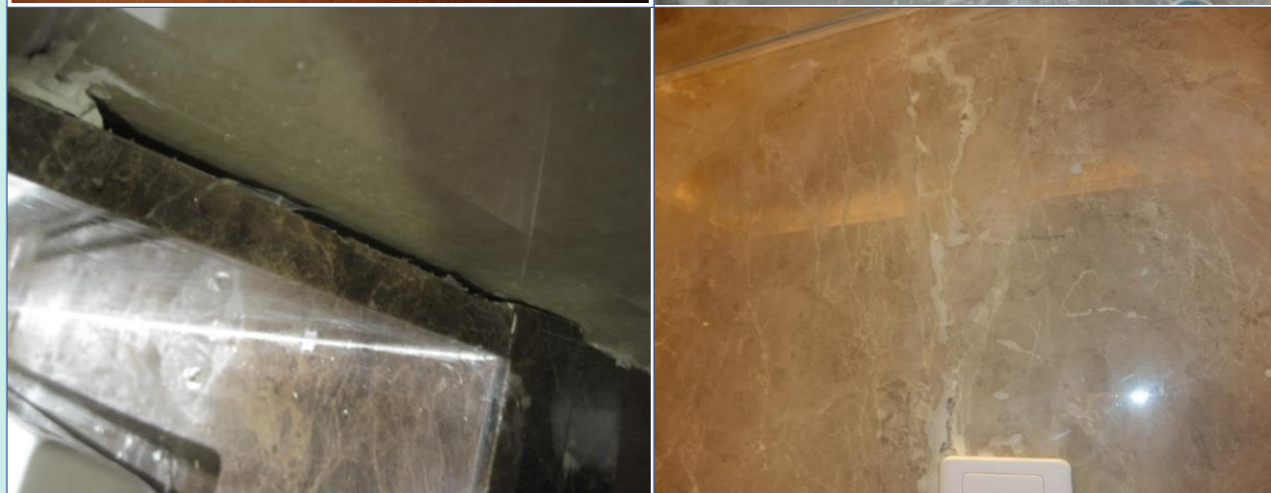
石材破损、断裂、缺棱掉角、色差、收口粗糙、污染
